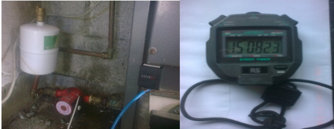
Figure 11 (a) Counter measuring on time Figure 11 (b) Watch measuring boiler cycle
